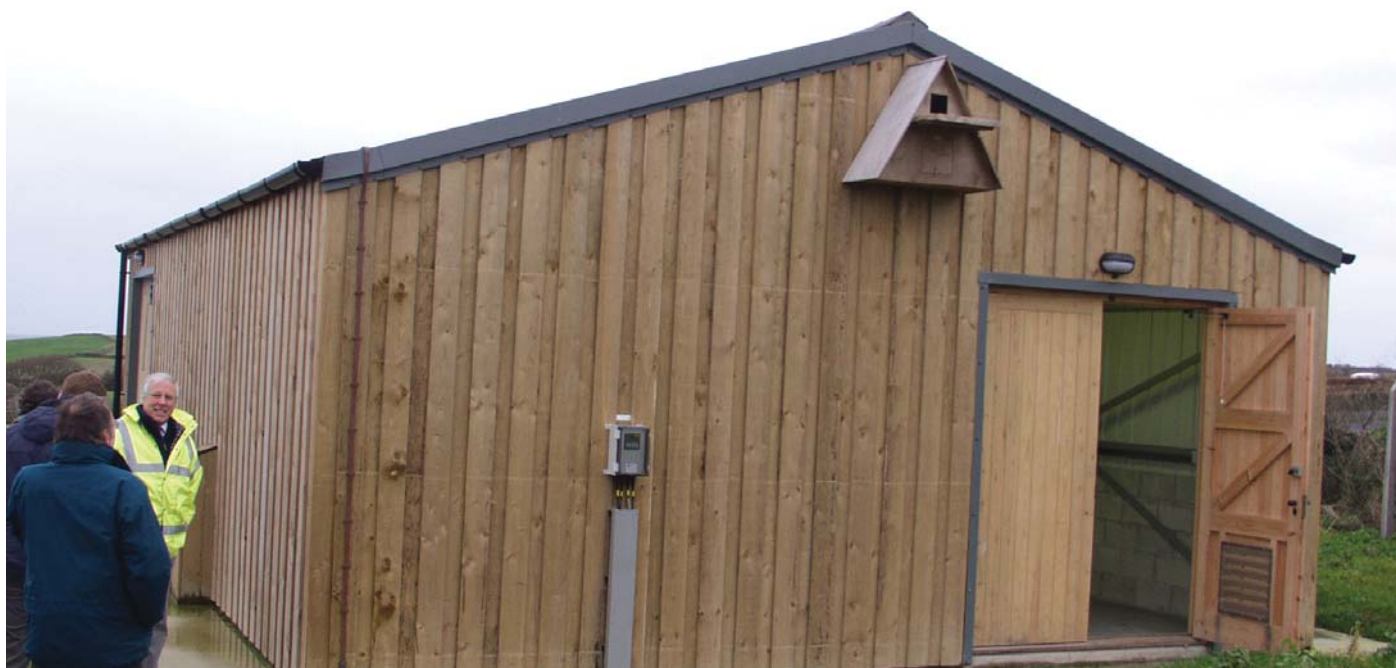
Small scale enhancement like this barn owl box on a South West Water building at Portscatho can be easily and inexpensively incorporated into the design of a development. Photo: Tim Warne
